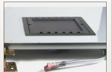
Installed Electrical/Voice/Data Box
